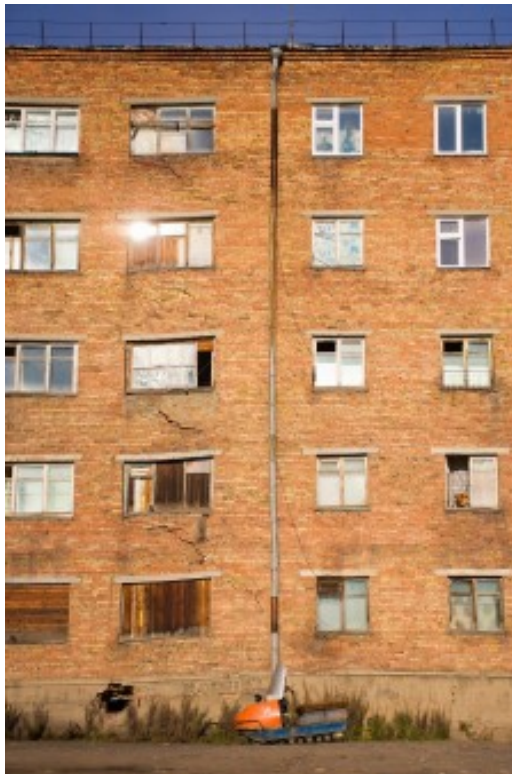
Building degrading from permafrost (Credit: Olga Dobrovidova)
